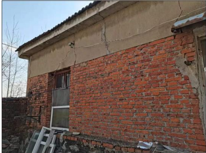
Figure 4. A Dilapidated House in Group G
