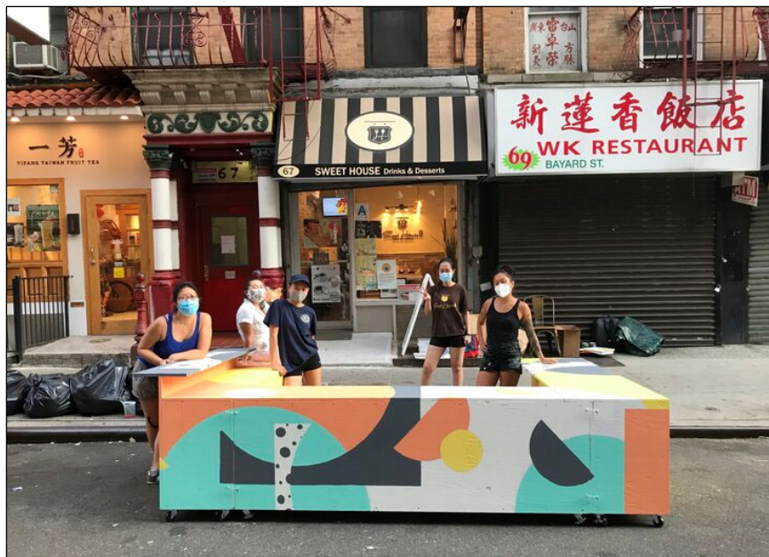
Figure 1. Think!Chinatown and women-led design studio A+A+A build new outdoor dining to support Sweet House Drinks & Desserts on 67 Bayard Street in their program Assembly for Chinatown. Photo by Think!Chinatown.
